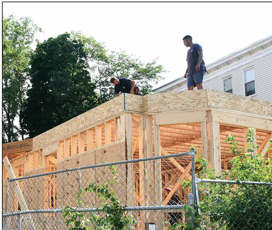
The three-decker on Church Street in Meetinghouse Hill was the company's first attempt at "building what was there." It got a great reception from neighbors who were happy he wasn't building "another spaceship" in the neighborhood
